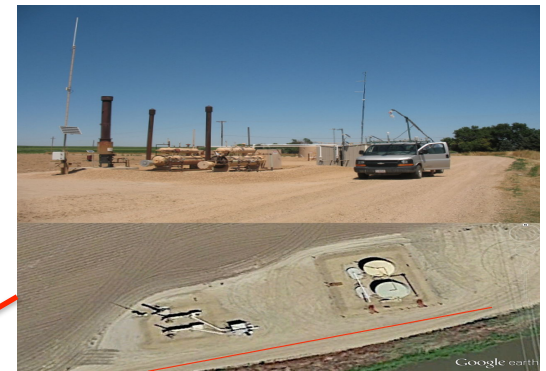
3. Oil and Gas Wells Conditions: These wells are located in a rural area in Weld County. Road traffic is limited at this location.
